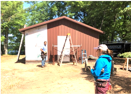
Maria Stone, Camp Manager, watching as the final sheets of siding are installed on the girl's cabin.
